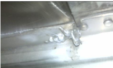
Roof patch repair damages top rail plainly visible from inside the unit.
